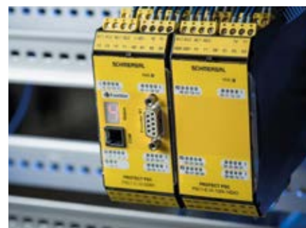
Fig. 5: The PSC1 system enabled cabling to be considerably reduced.
