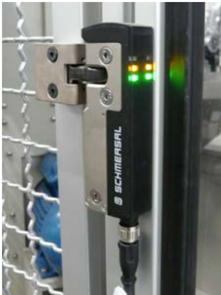
Fig. 1: The (safety) standard on the safety doors of the robot cells: the compact AZM40 solenoid interlock.
