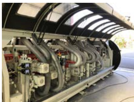
The processing machines on the Schroeder production line are secured with protective covers and solenoid interlocks.
